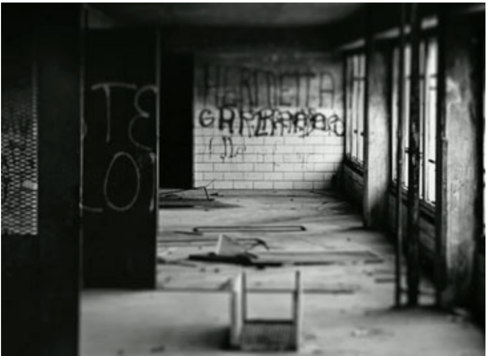
Figure 2, Interior Vandalism in a Pruitt Igoe apartment
