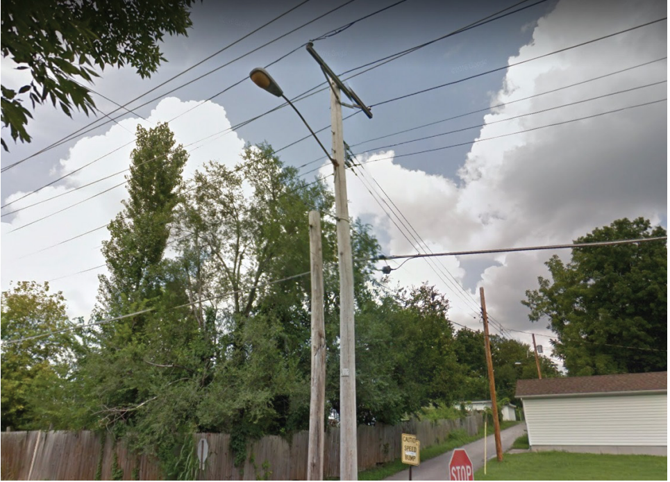
Existing Street Lights (Kingsland Avenue)
