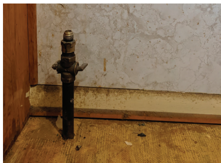
Starting from top to bottom: figures 6.21-6.22 Images depicting the dust and grease accumulated on the wall
