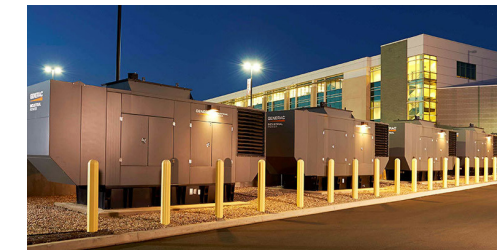
Image: (i45) Hospital Generators
