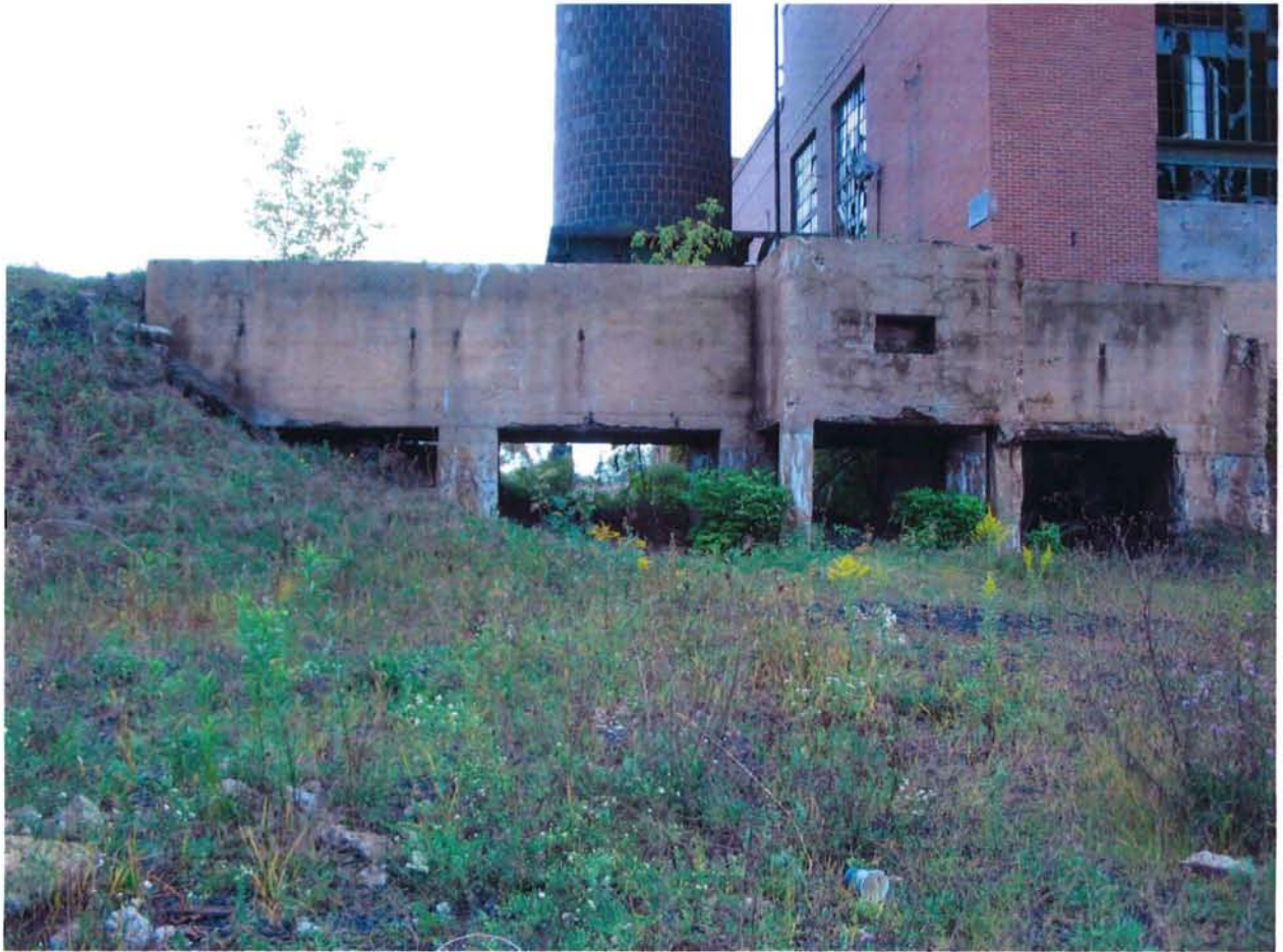
Figure 6.9 – View of concrete bridge concrete bridge that has fallen victim to the scars of weather and time. At one point in time, the bridge traversing the change in terrain had continued along the exterior elevation of the power plant. Currently, only a portion of the bridge and its supports remain. The following pictures represent further proof of the buildings’ extensive past.
